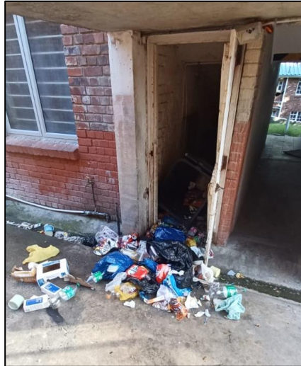
Figure 9. Problematic waste storage at Waterfall Barracks.
