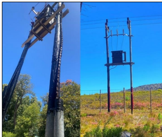
Figure 13. Examples of electrical infrastructure which poses an elevated risk of electrocution for baboons.
