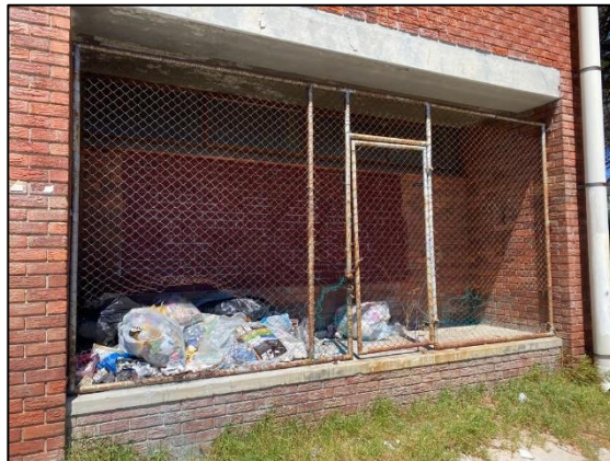
Figure 4. Waste cage at Jack's shop which requires repair.
